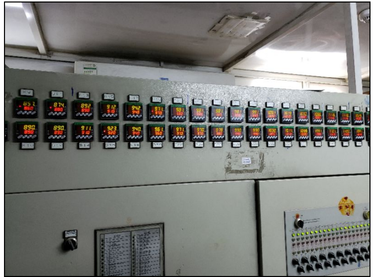
Burner cell thermostat 8 burners each
