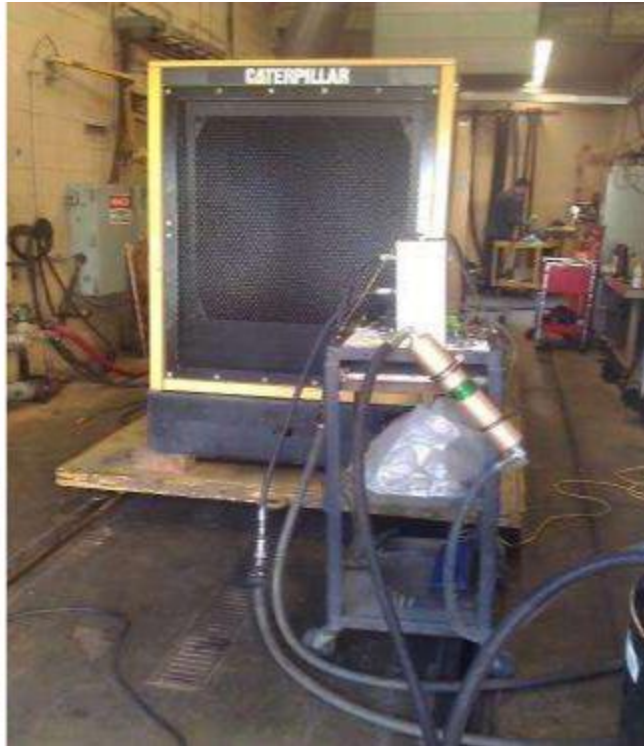
End view of engine with AIC meter and FFC
